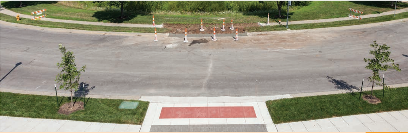
Work on the paved and stamped ADA crosswalk connecting Centerview and surrounding businesses to City Hall will be completed by Nov. 5, 2018.
