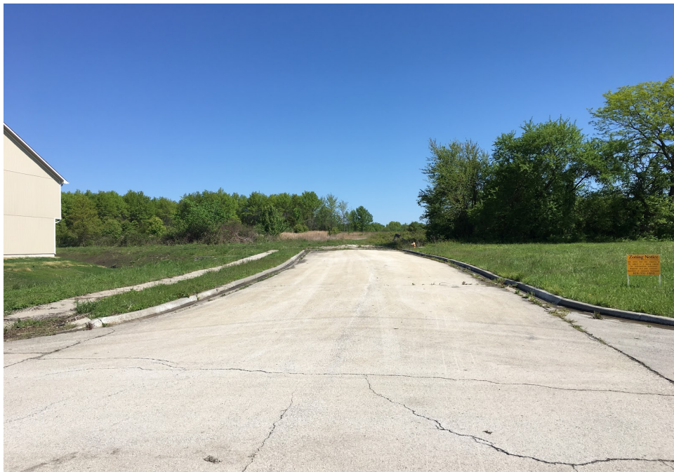
View looking north along Washington Street. Current road ends at the southern boundary of the subject property. (PUD zoning to the east, R-3A zoning to the west).
