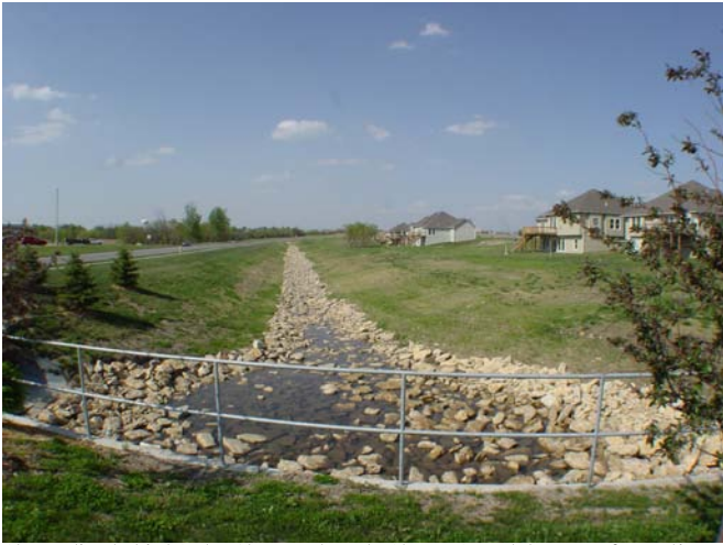
Channelized Third Order Stream at Eagle Glenn. Complete Loss of Aquatic and Terrestrial Habitat. Could be Improved With Native Grasses. (C)
