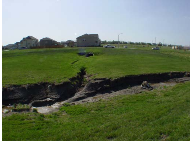
Pipe Outlet at Eagle Glen Without a BMP Has Caused Downcutting and Sedimentation. Fescue Grass Facilitates Surface Erosion and Provides Minimal Habitat
