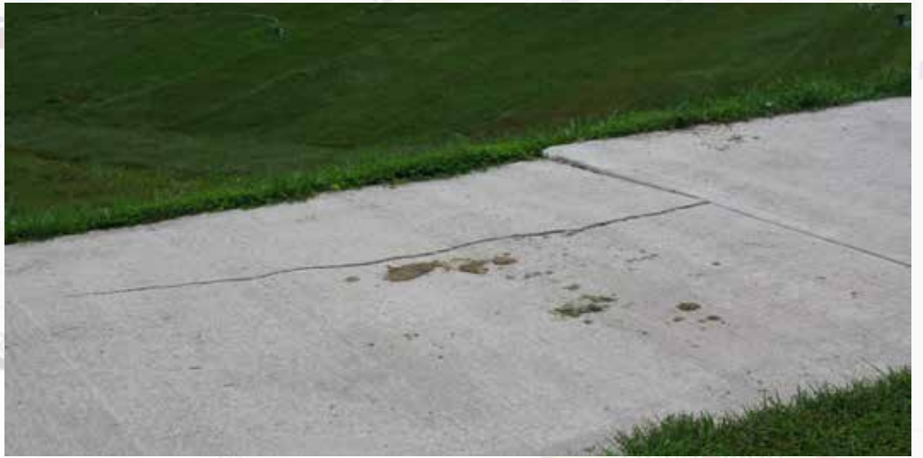
Potential subsidence of subgrade where trail is cracked and sinking slightly. Parks has already identified this for repair.
