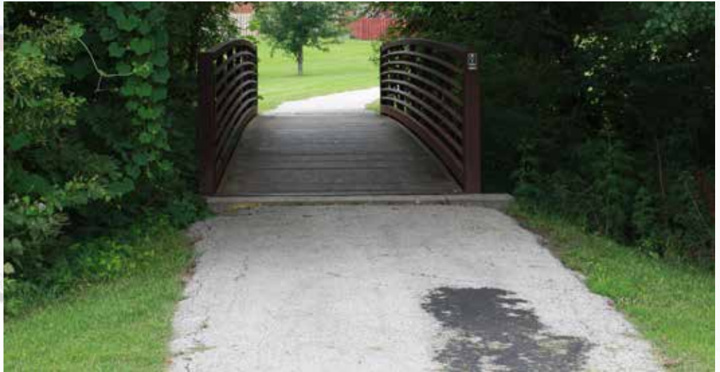
Good Parkway's asphalt is lifting over roots, cracking at culverts and sinking to make this elevation mismatch at a bridge abutment. Elevation adjustment already on Parks' winter project list. Recommendation: Replace Good Parkway asphalt trail segments with new cross-section standard.
