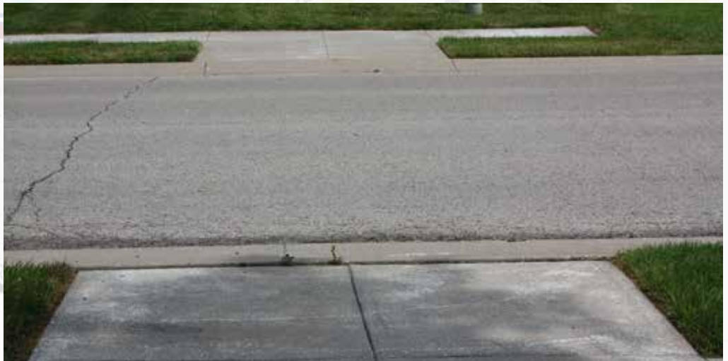
Trail currently ends at Shagbark without wayfinding direction. Hunt Midwest will be continuing trail to the north in the next year. Recommendation: provide temporary wayfinding to direct users to sidewalk on west side of Dean Ave.
