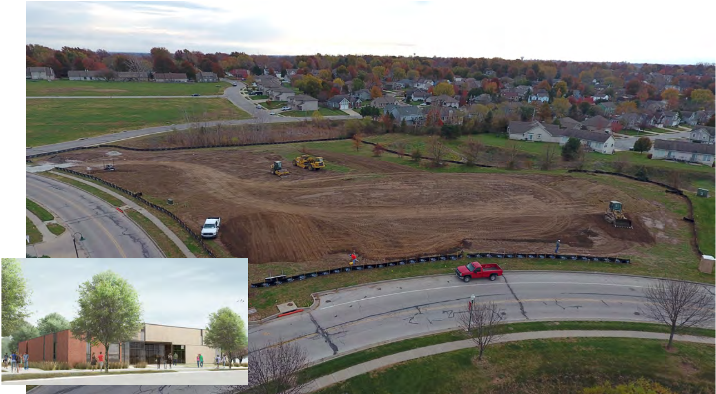
Contracts move dirt into place to begin building the foundation for Centerview, the City's new event space and community building. Once completed in the summer 2017, it will also be home to the Parks & Recreation Department.
