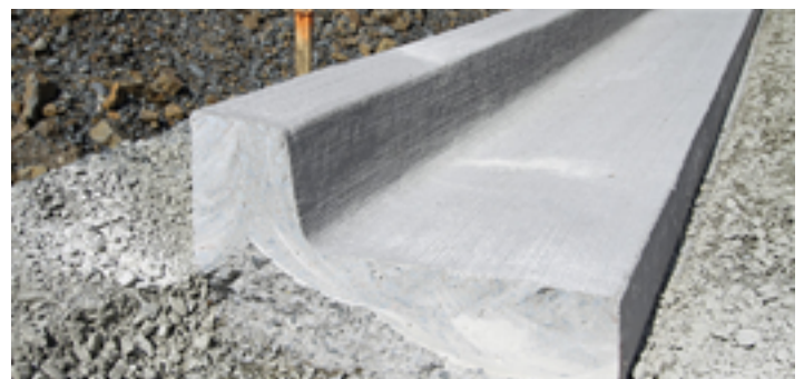
High back curb, which is being installed in the image above, is stronger and lasts longer than roll back curb.
