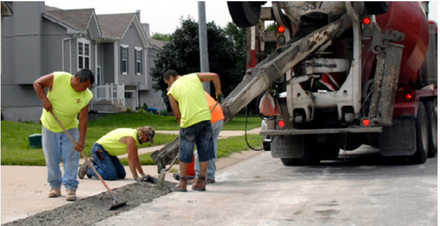
Contractors work to repair a row of roll back curb during the City's 2015 Curb Replacement Program.
