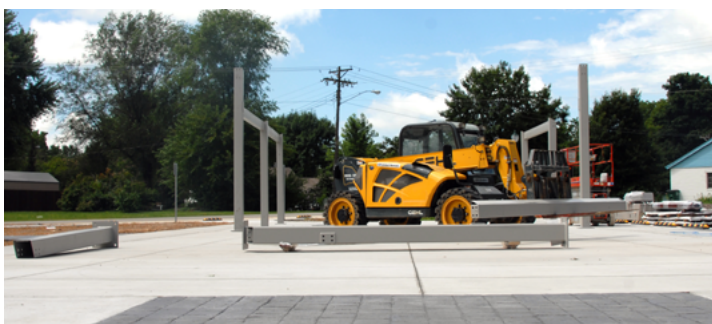
TOP: Steel beams frame the Depot shelter, which is under construction. BOTTOM: Crews move the steel beams into place on the new site.
